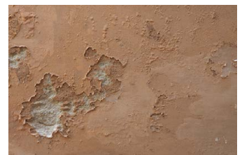
Damage to wall caused by flooding.
