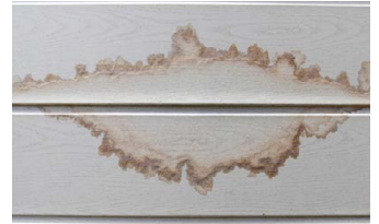
Water stained ceiling panels.
