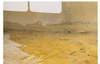
Wet area on floor and side of wall.
