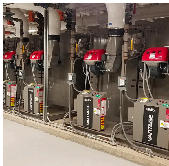
High Performance Hot Water Heating Plant Student Services Center Rockville Campus
