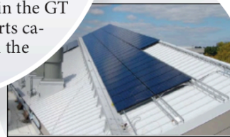
Rockville Campus Science Center Photovoltaic Array
